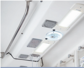
Cabin ceiling services panel
